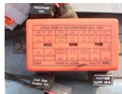
Feed Pump Fuse
