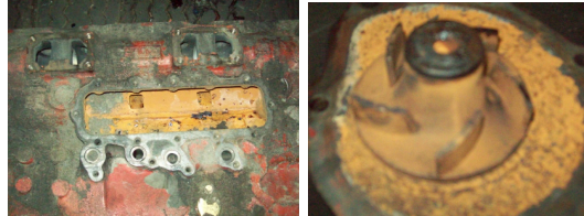
Engine block & Cooler plates with Heavy scale formation (Coolant additive not used in recommended ratio)
